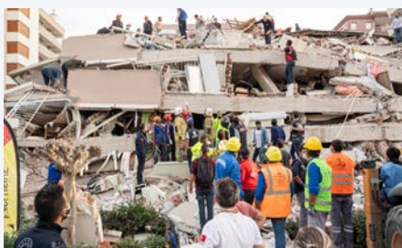
View of one of the collapsed buildings during the 2020 earthquake
