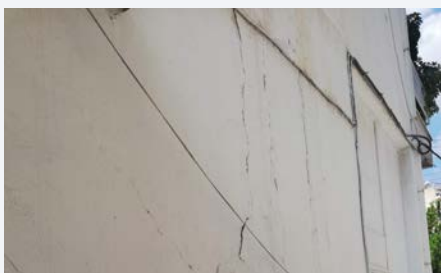
Cracks in structural elements of school buildings in Palaio Faliro after the earthquake in 2019
